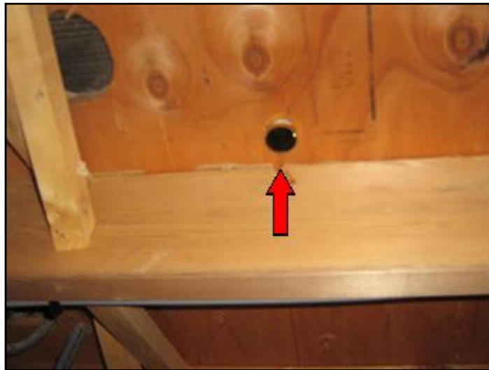
Poor termination of pan drain
