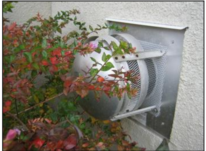
Too close to direct vent for fireplace
