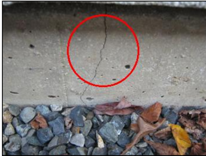
Typical foundation crack
